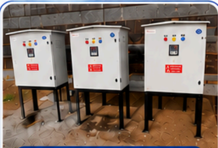
FEEDER PILLAR PANEL
