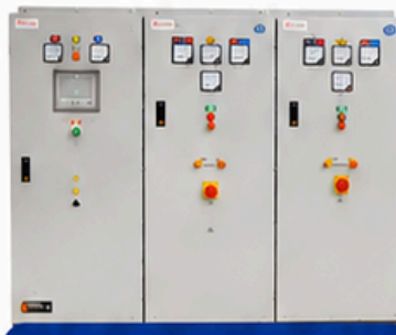
AC DB / SOLAR PANEL
